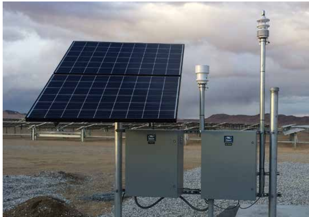
In addition to the standard measures, this meteorological station monitors precipitation. This station also includes a battery backup and PV-based recharging system to provide autonomous operation and ongoing data capture in case of power disruption.
